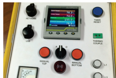
Electronic control box with data logger for regulating temperature
